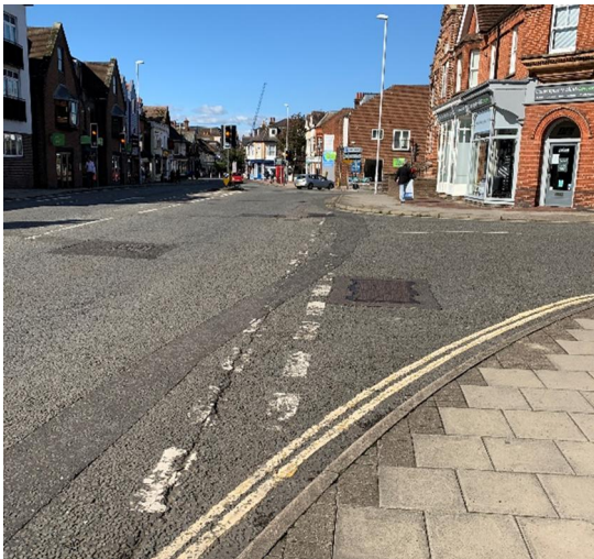
Wide side road crossing at Barttelot Road
